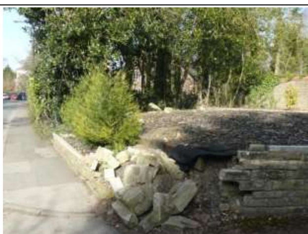
Photograph 26: Damaged Stone Boundary Wall and Tarmac Patch Repairs
